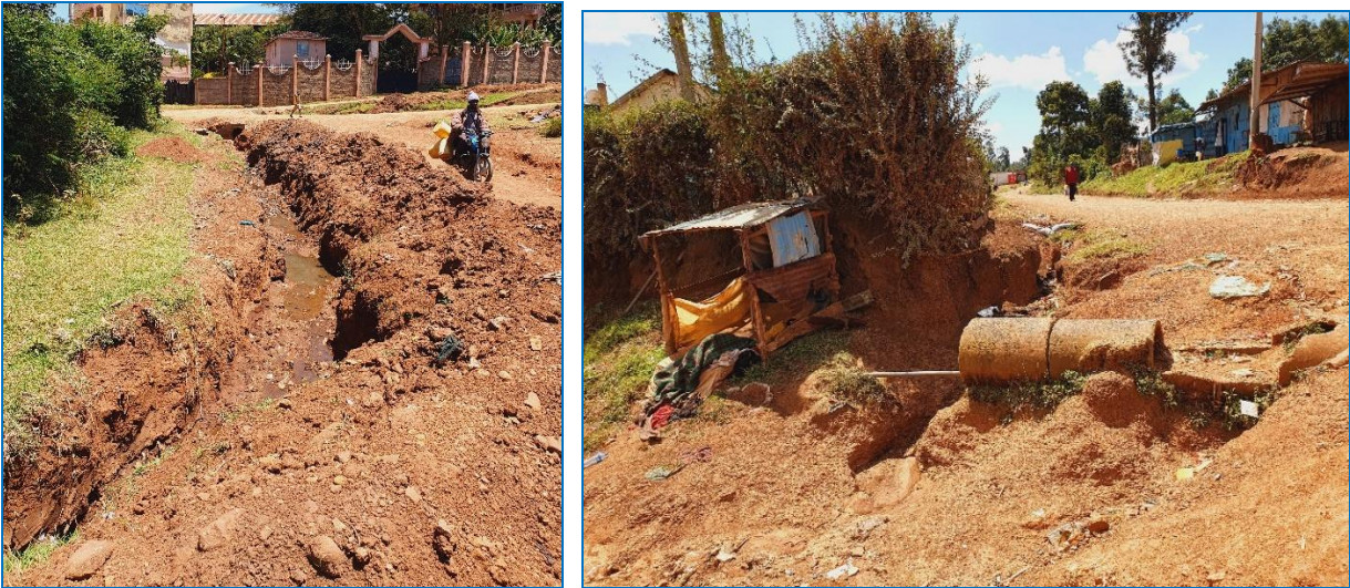
Plate 16: Poor storm water drainage channels
