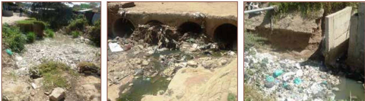
Photo 8.2: Solid waste dumped on Open Storm Water Drains
