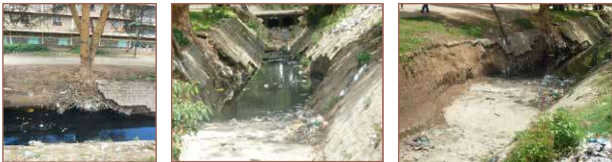
Photo 8.3: Patches of the Stone pitched Kakia Valley Drains Washed Away
