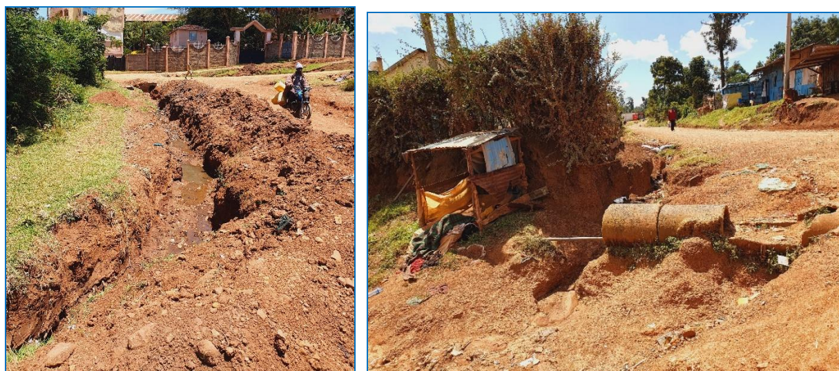
Plate 16: Poor storm water drainage channels
